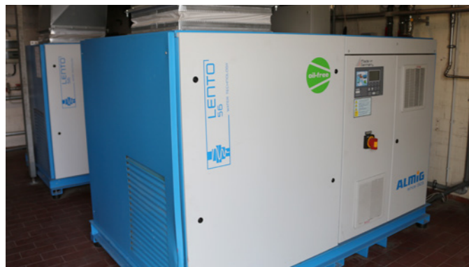
Bad Meinberger relies on oil-free water-injected screw compressors of the LENTO series from ALMiG.
